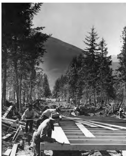
Figure1. House Building, New Denver, B.C., 1942, Leonard Frank photos, Alex Eastwood Collection, Nikkei National Museum, 1994.69.4.21.
