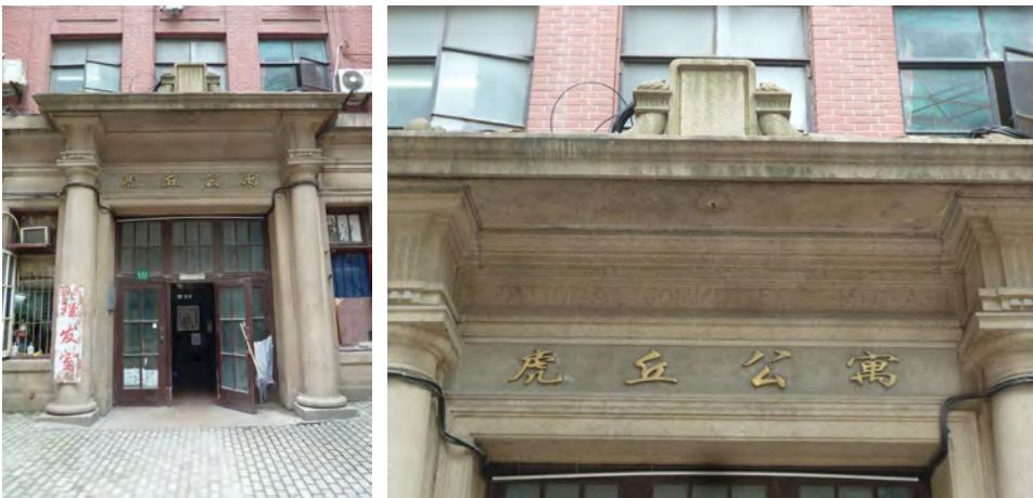
Fig. 1 Entablature of YMCA National Headquarters Shanghai. Shattuck & Hussey, architects, 1921 (l). Detail shows faint outline of the words 'NATIONAL COMMITTEE Y.M.C.A.', and the YMCA torches above surrounding a shield, which may have held the international 'Y' triangle (r). Photographs by Anne Warr, May 2015.
