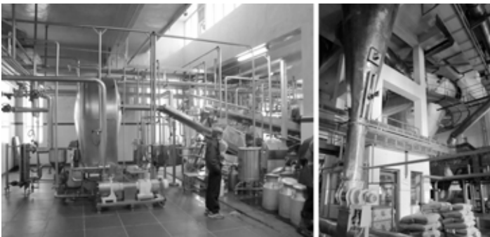
Figure 1. Interior views showing milk processing area and multistorey powder-plant with natural light and ventilation. Photographs by the author.
