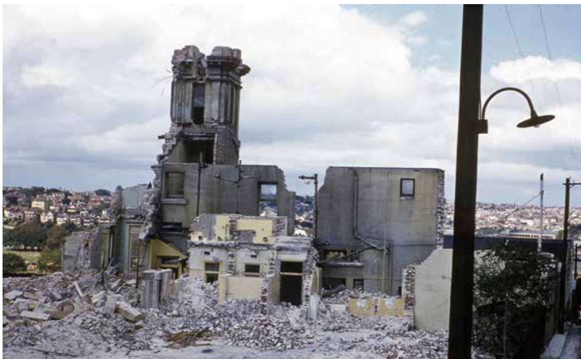
FIGURE 7 The partially demolished Kinneil, with its east tower still almost standing, 1971. (Photo by Robert Walker. City of Sydney Archives).
