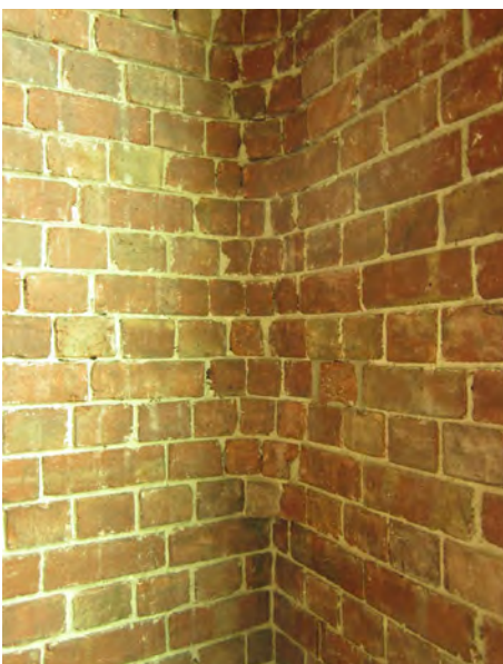
Fig. 3 St Vincent's Hospital 1905 building, stairwell with cement render removed. Photograph by Karen Daws, 2015.
