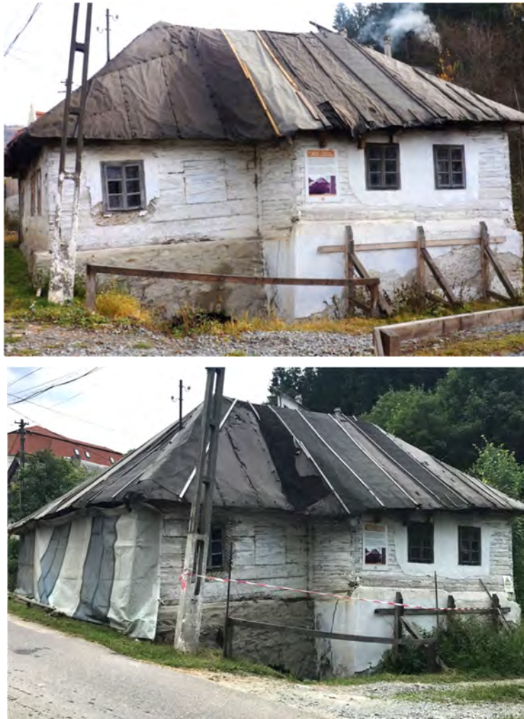
Figure 3. House no. 301. The roof is covered for protection and timber posts support the exterior wall. The finish that has degraded over time is visible around the windows and the base. Top image: 2014, Bottom image: 2017 (Photographs by Alexandra Florea).
