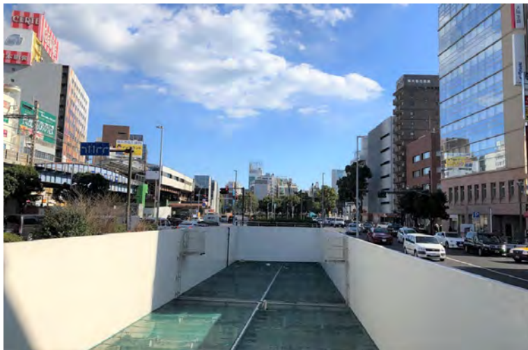
Figure 16. Completed open-cut motorway on the ground level in 2019 (Photograph by Toshio Taguchi).
