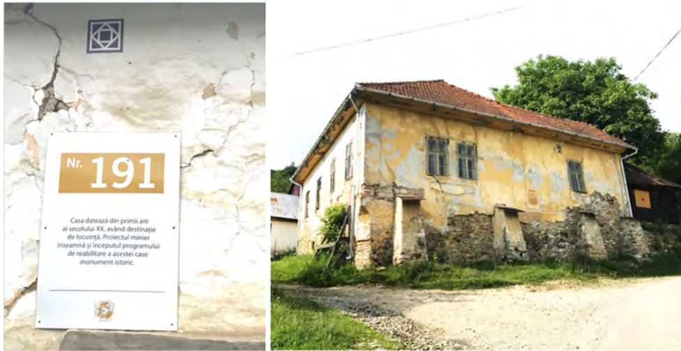
Figure 5. Examples of derelict buildings that have been labelled as proposed for restoration once the mining project starts (Photographs by Alexandra Florea).
