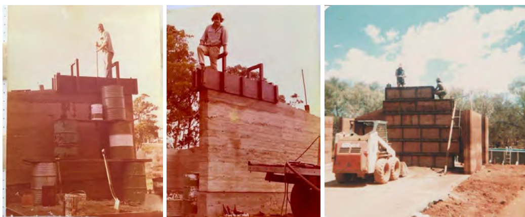
Figure 4. (A) Tom Roberts during the construction of the Shed, at Cape Mentelle Winery Estate, Middleton Formwork system 1976; (B) G. Hohnen during the construction of the Shed, at Cape Mentelle Winery Estate, Middleton Formwork system 1976; (C) The new formwork system. Courtesy of G. Hohnen.
