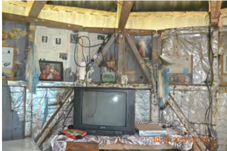
Fig. 9. Interior of Kaho's aid house showing no ceiling and soffit linings, author September 2013
