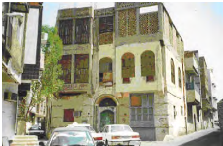
Fig. 4. Hybrid architecture in Makkah. Note the use of concrete in the large opening that was formerly covered by a roushan .
